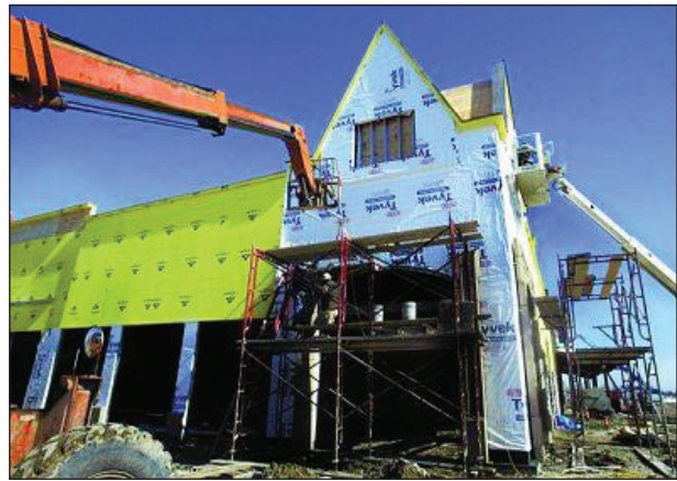
Construction continues on what will be the first L.L. Bean store in the Midwest at The Arboretum of South Barrington, a new shopping center scheduled to open this fall. (Michelle Lohmann/Staff Photographer)
